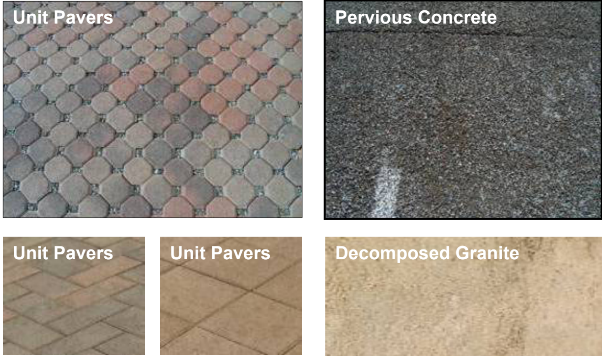
Figure 4: Pervious Pavement used at Headquarters
